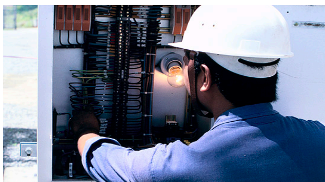
A worker in Caracas repairs the grid, helping to ensure reliable service.
